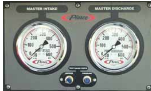
MASTER DISCHARGE PRESSURE GAUGE (RIGHT)
