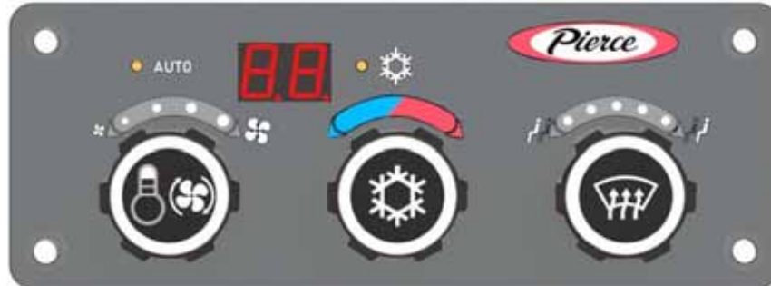
Figure 4-6: HVAC Control Panel
